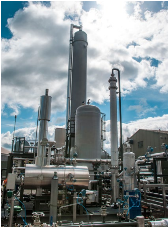
TEG Biogas Drying at Groot Zevert Vergisting
