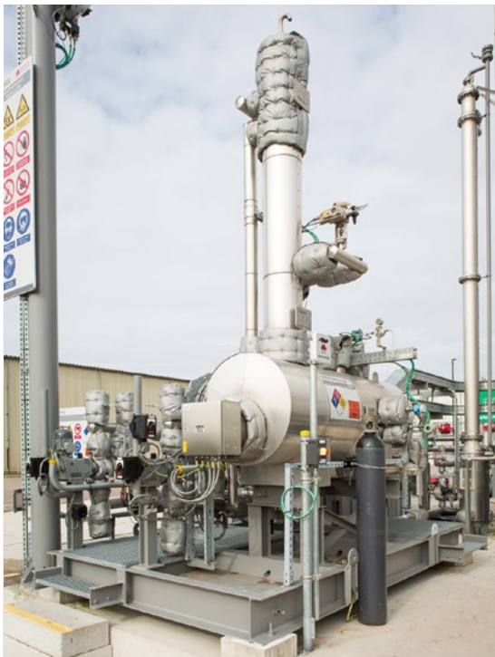
TEG Biogas Drying at HVC Middenmeer
