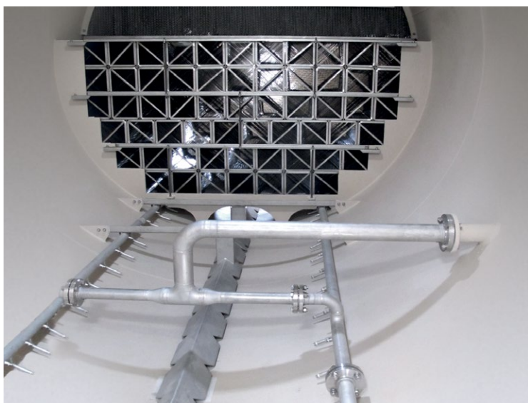
Coalescing Plate Packs with Sand Jetting
