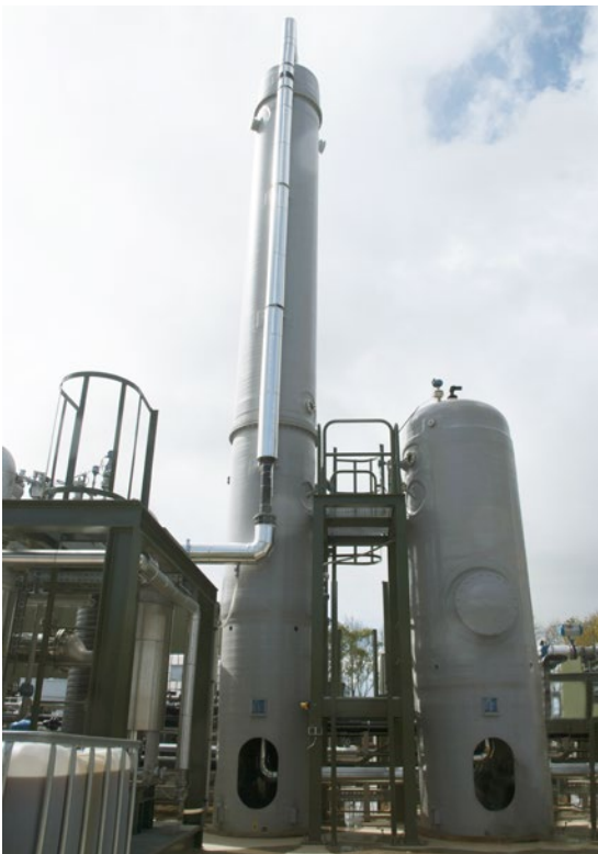
Picture 2 - Regenerative LAMINOL® installation
