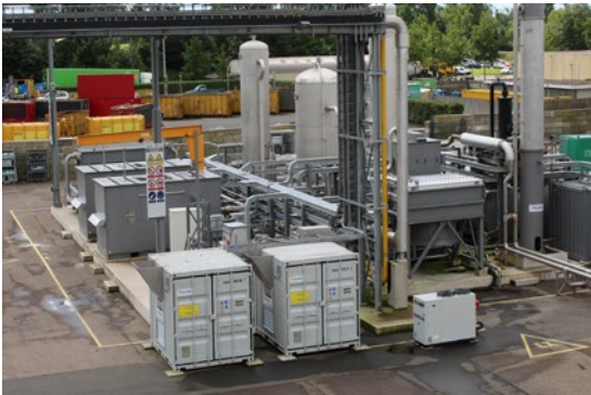
Picture 1 - Scavenger based LAMINOL® installation
