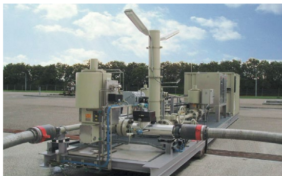
Middelie, NAM, Gas Production 2 Skids – the Netherlands
