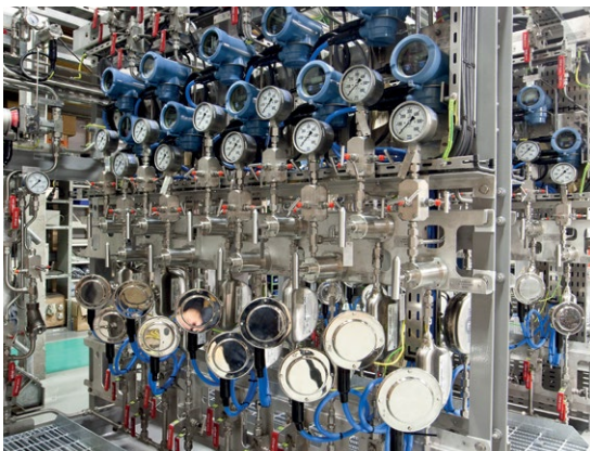
Turret Chemical Distribution Package
