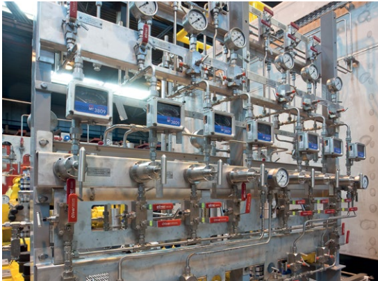
Manual Operated Distribution System on a Chemical Injection Package
