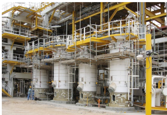
Desiccant Dehydration - Dolphin Onshore Gas Plant Project
