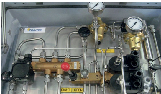
Control Panel for Natural Gas Driven Actuators
