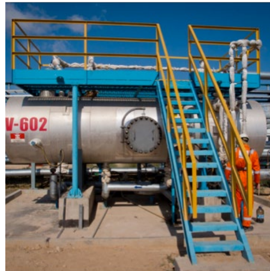
Induced Gas Flotation Vessel
