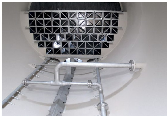
Coalescing Plate Packs with Sand Jetting
