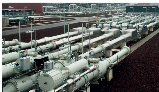
Pneumatic Actuated Valves in a Process Line
