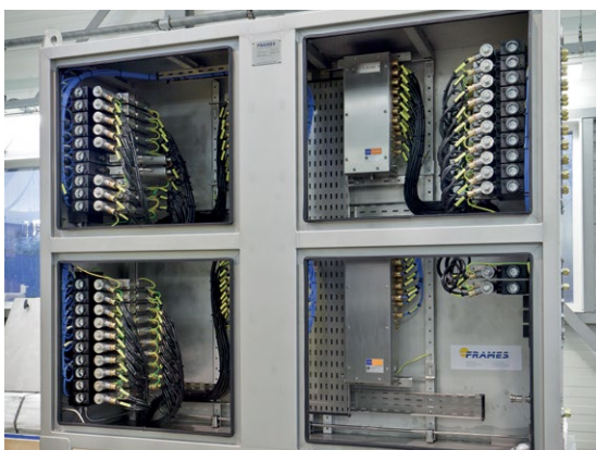
Local Control Panel
