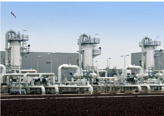
Gas Dehydration Towers
