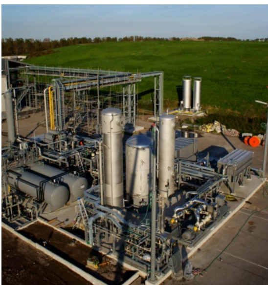
Overview green gas installation HVC Middenmeer
