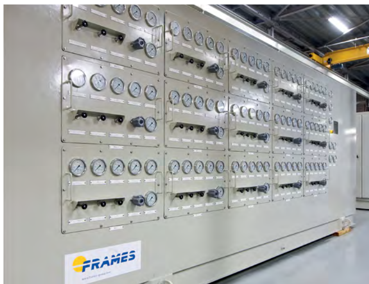
Frames Multi Wellhead Control Panel
