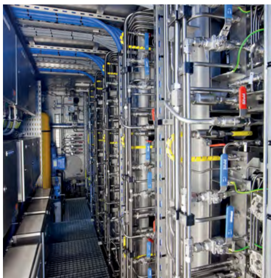
Walk-in Type Wellhead Control Panel
